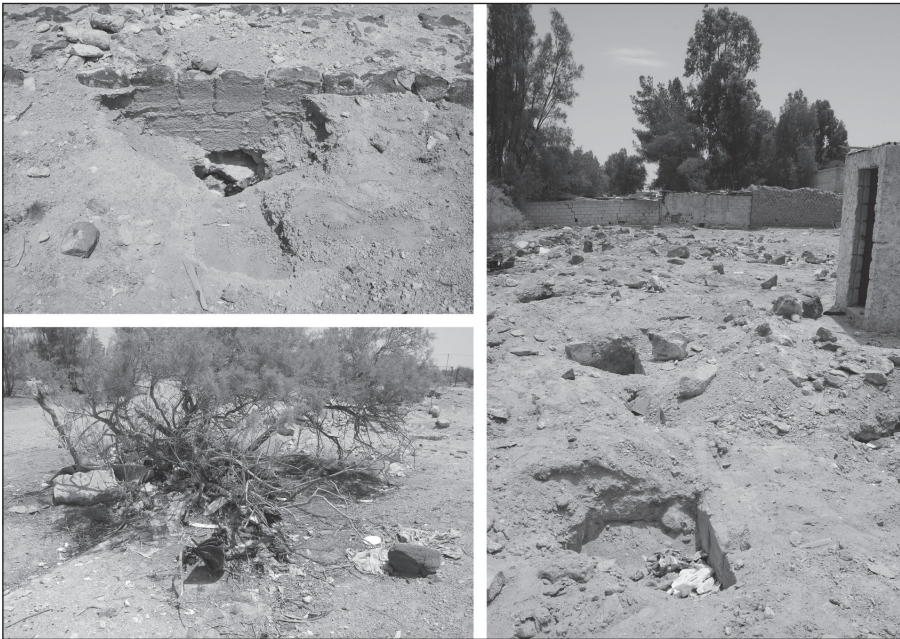
21. Examples of the current state of preservation of the wall of the reservoir-enclosure outside the reserve (AASRP 2015).
